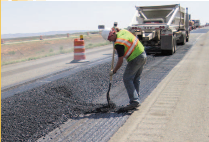
The GlasGrid System allowed the contractor to make repairs quickly using temporary, one-day lane closures.
